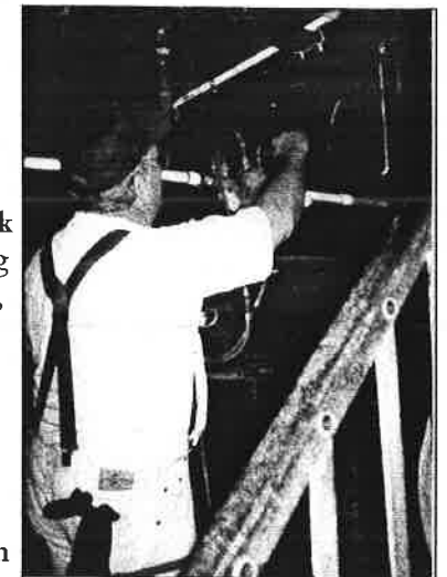
Many backflow preventers are in hard to reach places - making it even harder to repair
