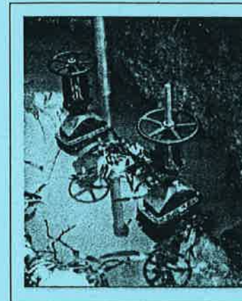
Is there a backflow preventer here?
